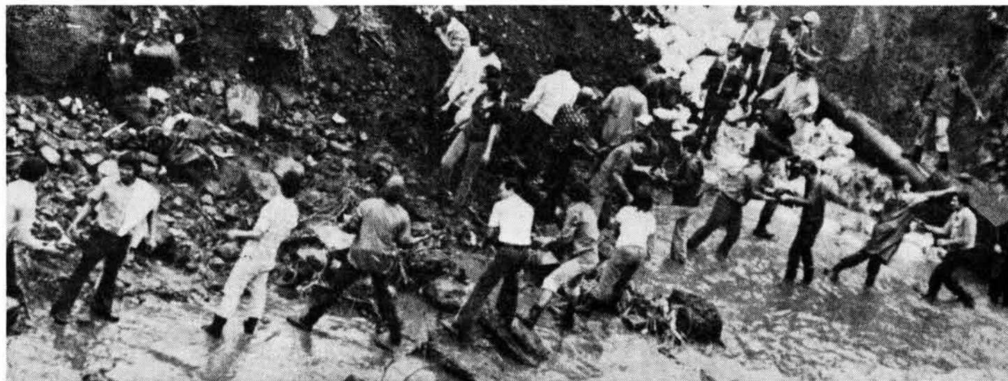
Volunteer workers building dikes in Managua. Floods caused some $200 million in damage and left tens of thousands homeless. Barricada
