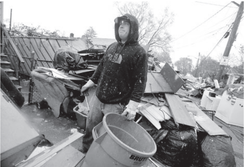
Matthew Czirr clears debris from his grandmother’s home in New Dorp section of Staten Island, N.Y., Nov. 7. Snow falls as another storm brews with evacuation urged in some areas.
